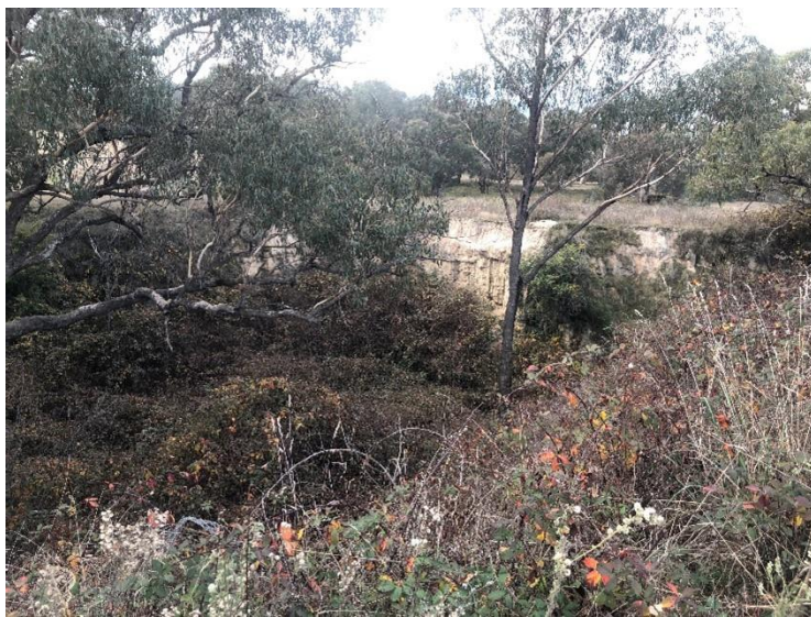
Figure 10: Frying Pan Creek tributary blowout on Tarana Road.
